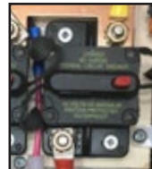
80 Amp Charger Output Breaker
