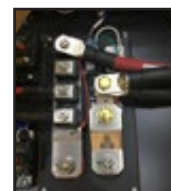
Battery Shunt Fuse
