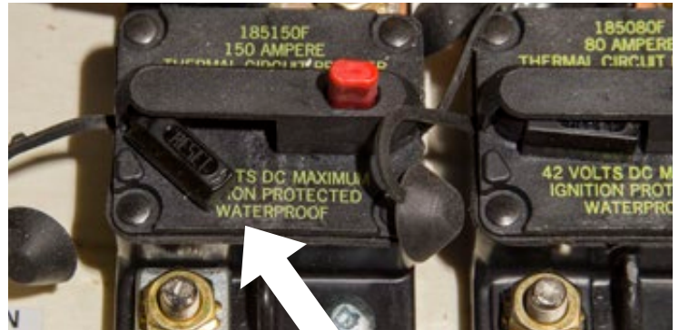
ARM DOWN INDICATES TRIPPED BREAKER
