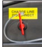
Charge Line Disconnect (red key)
