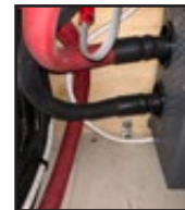
Inverter DC Output
