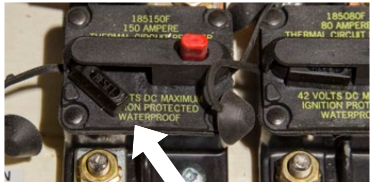
ARM DOWN INDICATES TRIPPED BREAKER
