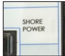
Distribution Panel Shore Power Breaker
