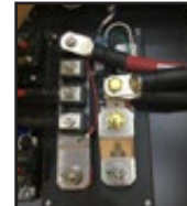
Battery Shunt Fuse
