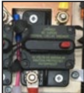
80 Amp Charger Output Breaker
