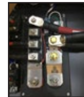
Battery Shunt Fuse
