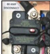
80 Amp Charger Input Breaker
