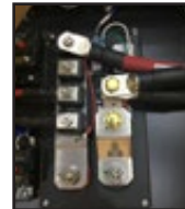
Battery Shunt Fuse
