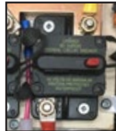
80 Amp Charger Output Breaker
