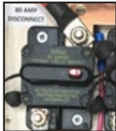
80 Amp Charger Input Breaker
