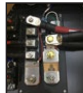
Battery Shunt Fuse
