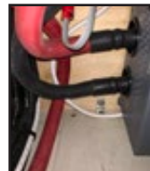
Inverter DC Output
