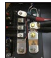
Battery Shunt Fuse
