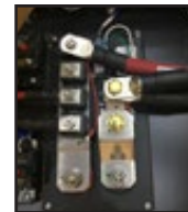
Battery Shunt Fuse
