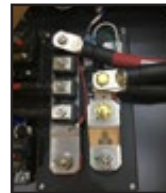
Battery Shunt Fuse
