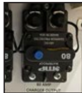
80 Amp Charger Output Breaker
