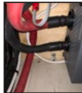
Inverter DC Output
