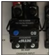
80 Amp Charger Input Breaker
