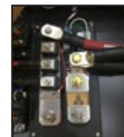
Battery Shunt Fuse
