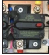
80 Amp Charger Output Breaker
