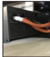
Inverter DC Output
