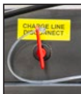
Charge Line Disconnect (red key)
