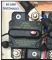
80 Amp Charger Input Breaker
