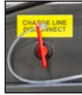
Charge Line Disconnect (red key)
