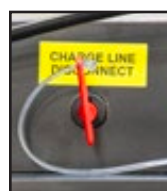
Charge Line Disconnect (red key)
