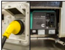
Shore Power or Generator
