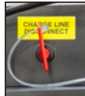
Charge Line Disconnect (red key)
