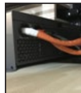
Inverter DC Output
