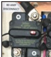
80 Amp Charger Input Breaker
