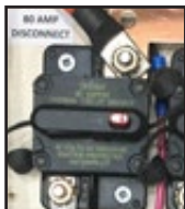
80 Amp Charger Input Breaker
