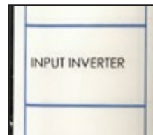
Distribution Panel Input Inverter Breaker
