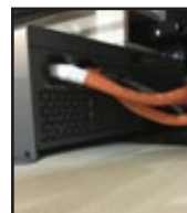
Inverter DC Output
