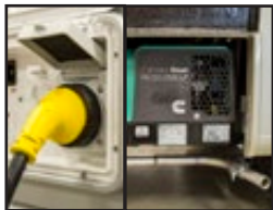
Shore Power or Generator
