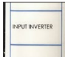
Distribution Panel Input Inverter Breaker
