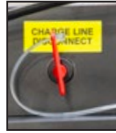
Charge Line Disconnect (red key)
