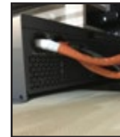
Inverter DC Output
