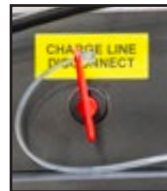
Charge Line Disconnect (red key)
