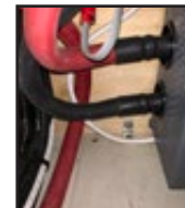
Inverter DC Output
