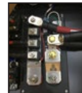
Battery Shunt Fuse
