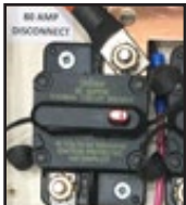
80 Amp Charger Input Breaker
