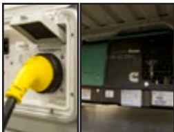
Shore Power or Generator
