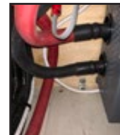
Inverter DC Output
