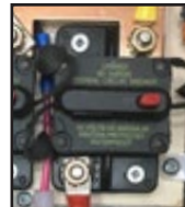
80 Amp Charger Output Breaker
