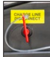
Charge Line Disconnect (red key)
