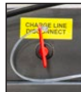
Charge Line Disconnect (red key)
