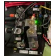
Battery Shunt Fuse
