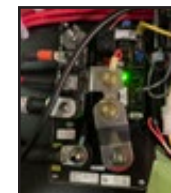
Battery Shunt Fuse
