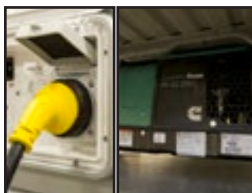
Shore Power or Generator
