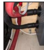
Inverter DC Output
