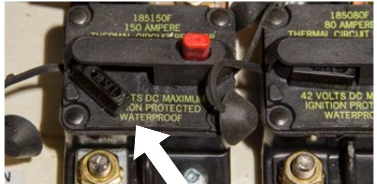
ARM DOWN INDICATES TRIPPED BREAKER
