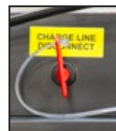
Charge Line Disconnect (red key)
