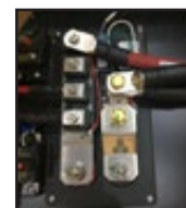
Battery Shunt Fuse
