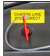
Charge Line Disconnect (red key)
