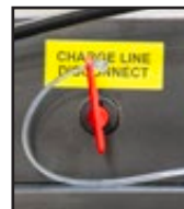
Charge Line Disconnect (red key)
