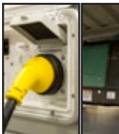
Shore Power or Generator
