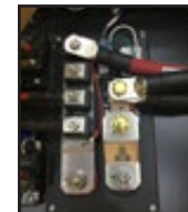
Battery Shunt Fuse
