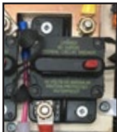
80 Amp Charger Output Breaker
