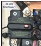
80 Amp Charger Input Breaker
