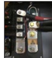
Battery Shunt Fuse
