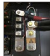
Battery Shunt Fuse
