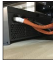
Inverter DC Output
