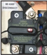
80 Amp Charger Input Breaker
