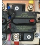
80 Amp Charger Output Breaker
