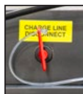
Charge Line Disconnect (red key)
