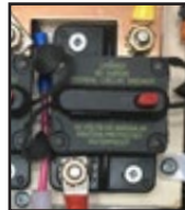
80 Amp Charger Output Breaker
