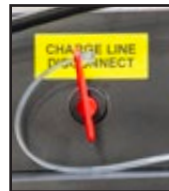
Charge Line Disconnect (red key)
