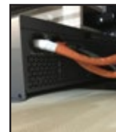
Inverter DC Output
