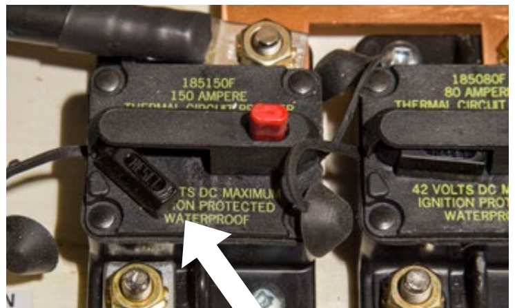
ARM DOWN INDICATES TRIPPED BREAKER
