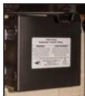
Automatic Transfer Switch
