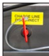
Charge Line Disconnect (red key)
