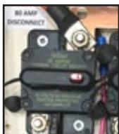
80 Amp Charger Input Breaker
