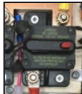
80 Amp Charger Output Breaker
