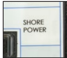
Distribution Panel Shore Power Breaker
