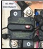
80 Amp Charger Input Breaker
