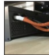
Inverter DC Output
