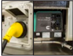
Shore Power or Generator
