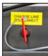
Charge Line Disconnect (red key)
