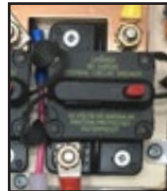
80 Amp Charger Output Breaker
