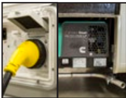
Shore Power or Generator
